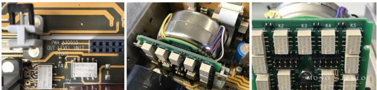
Location of one Nagra transformer board on the main board (left), left channel Nagra transformer board (middle) and switching relays (right).
